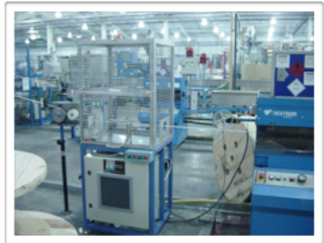
Six systems installed operating on Propane
