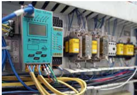
Safety PLC Upgrade
